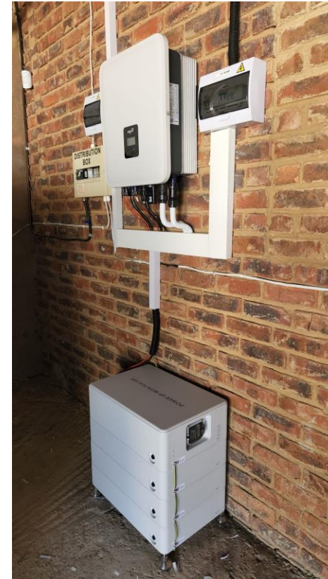
Solar inverter & battery
