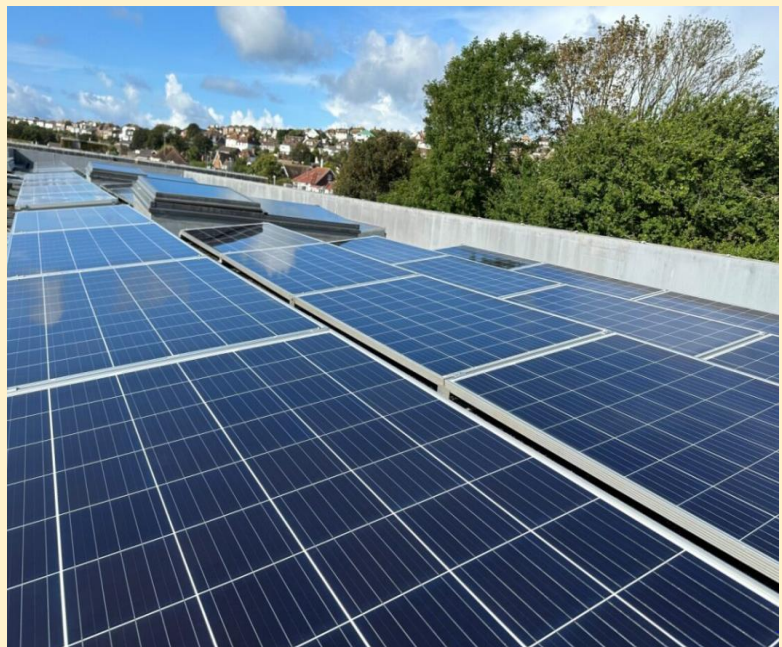
BHESCo solar power at Saltdean Primary School
