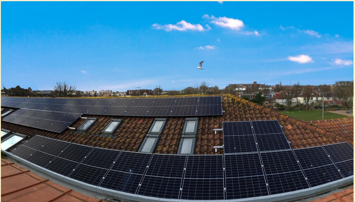
Solar panels installed at Brunswick Primary School through BHESCo's 2019 Share Offer
